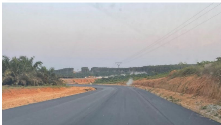
Photos One and Two | New Highway Under Construction and High Voltage Transmission Lines (southern Mining Permit boundary)
